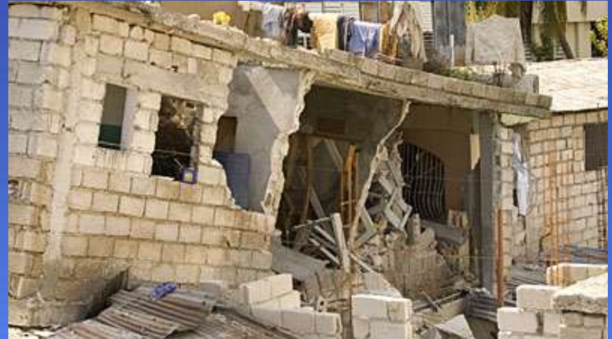
Poor concrete frame house
