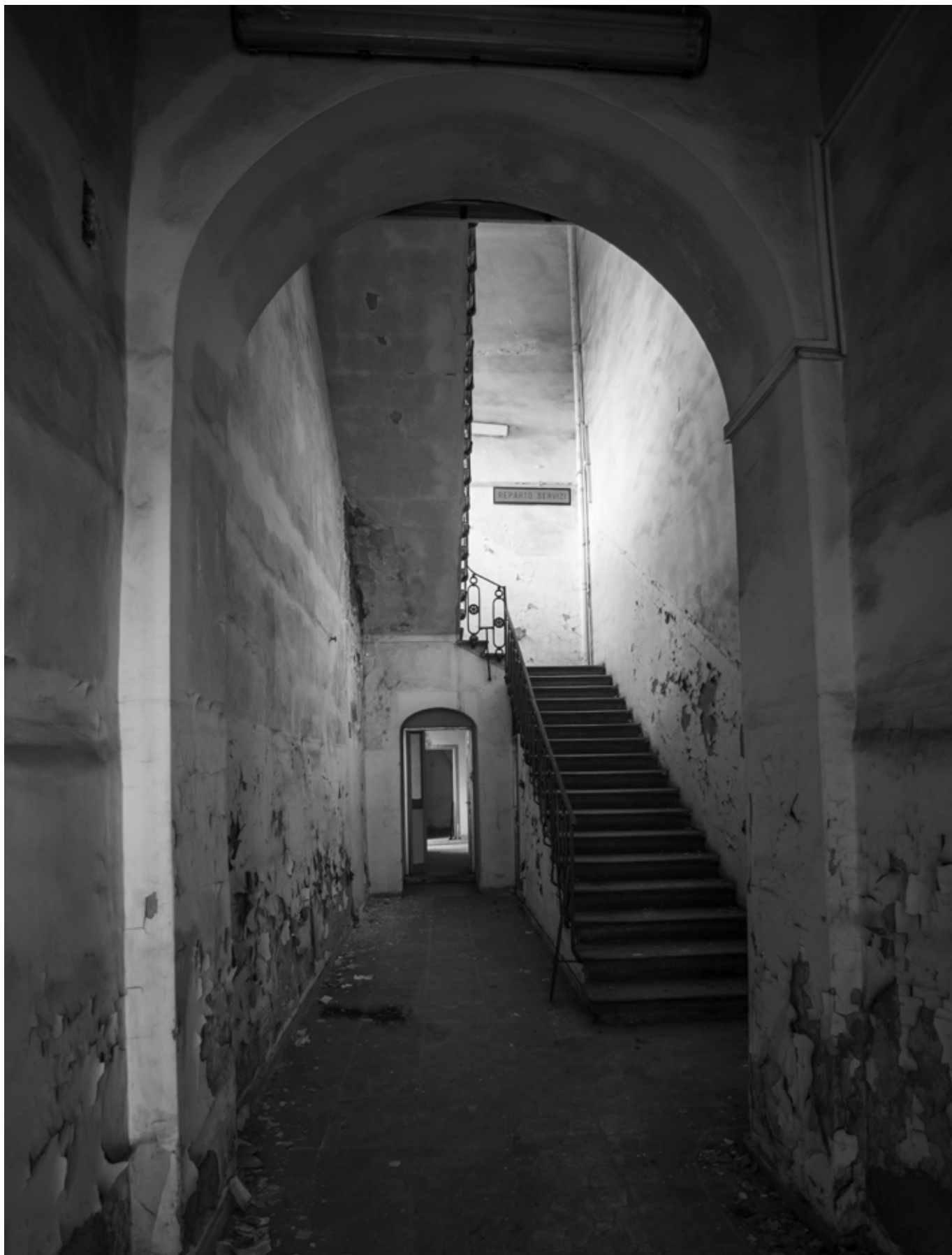
Vista interna / Inside view
