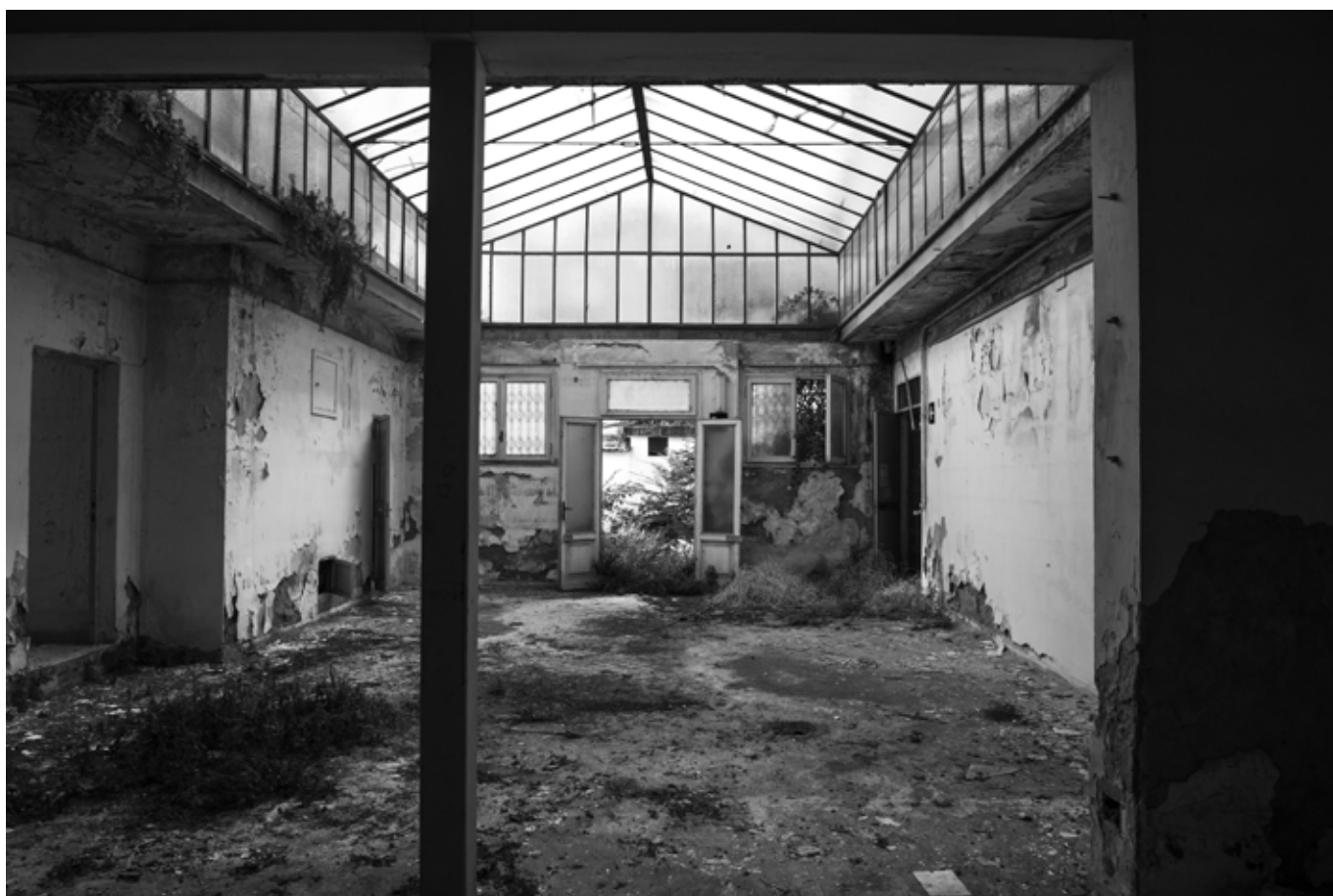
Vista interna / Inside view
